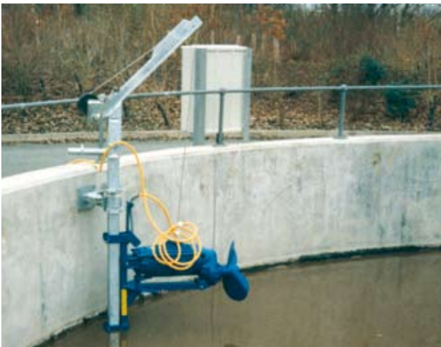
Submersible mixer GTWSI 1040 in a sludge basin of a sewage plant
